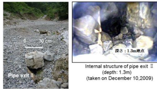
Fig.1 Exposed pipe exit II at the torrent bed material due to its scouring on October 24, 2008 and its internal structure
