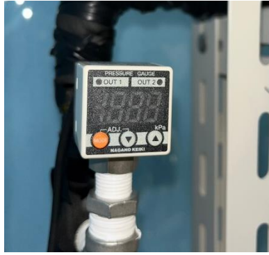
Figure 3-25 Photo of digital pressure gauge
