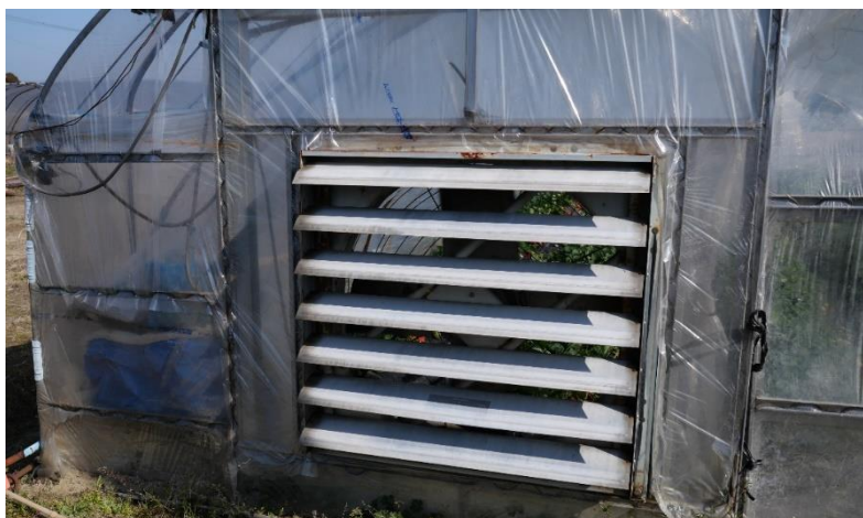
Figure 3-4 (b) Ventilation fan
