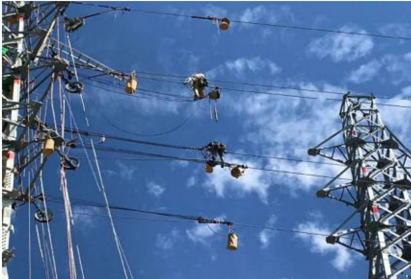
Fig.2.3 Electric wire embarking in the air
