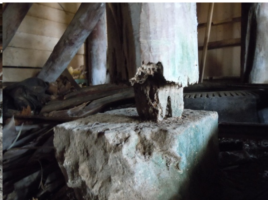
Photo.3-14 Harms by termite
