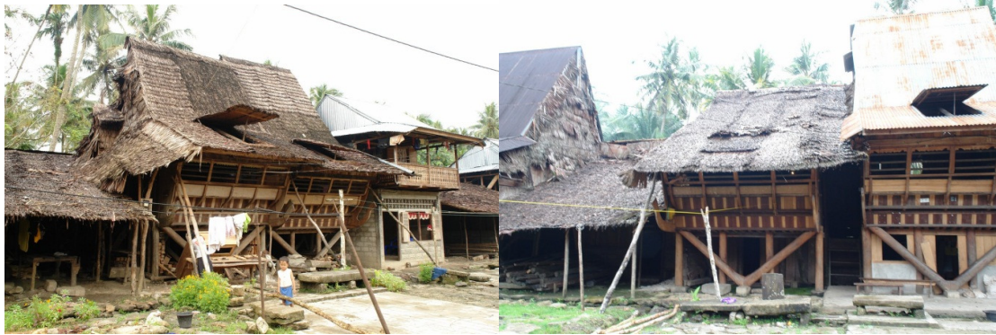
Photo.1-9 Traditional houses damaged by earthquakes leaned to front
