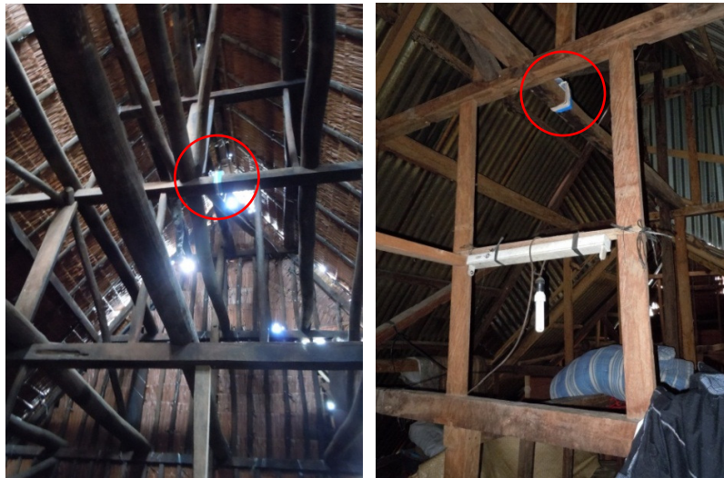
Photo.4-3 Arrangement of the sensors inside roof frame
