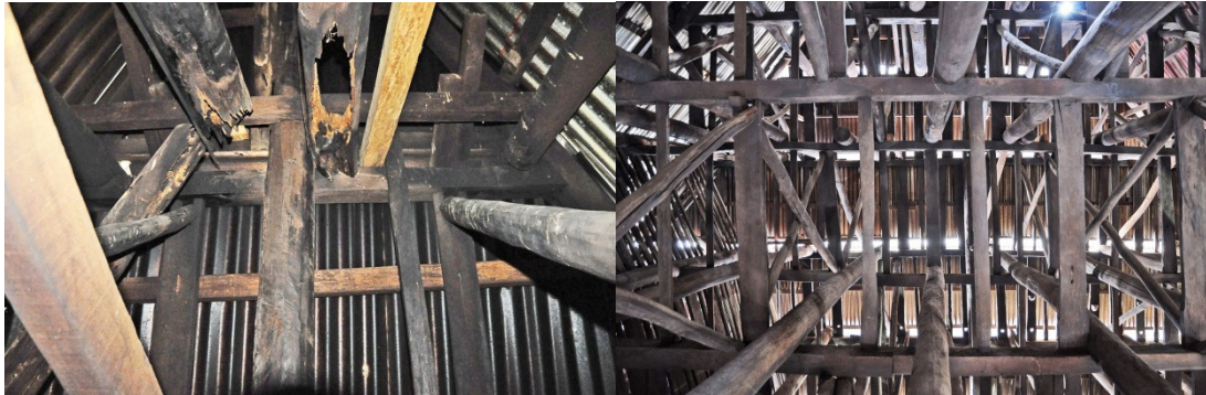
Photo.3-5 Harms by termite and roof frame
