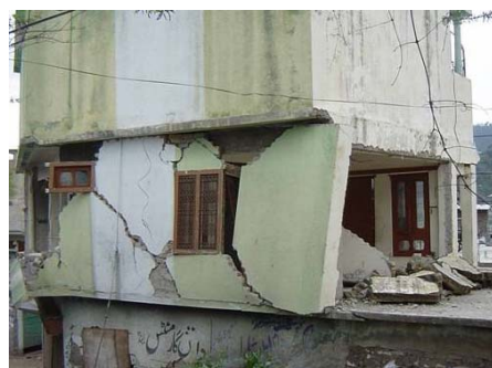
Fig. 81 Diagonal cracks on actual building in Pakistan
