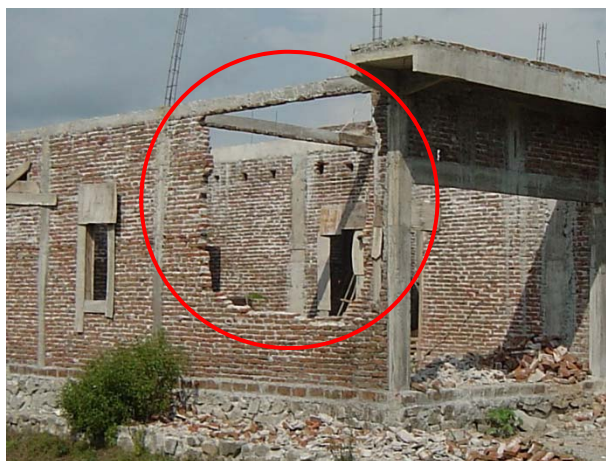
Fig.61 Damaged house in Yogyakarta after 2006 Central Java Earthquake
