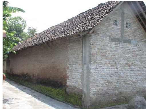
Fig.27 A variety of shapes and deterioration levels
