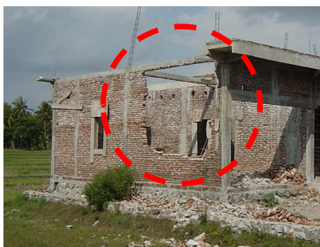
Fig. 85 Out-of-plane failure on actual building in Indonesia
