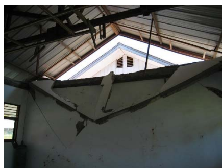
Fig. 89 Out-of-plane failure of gable wall on actual building in Indonesia
